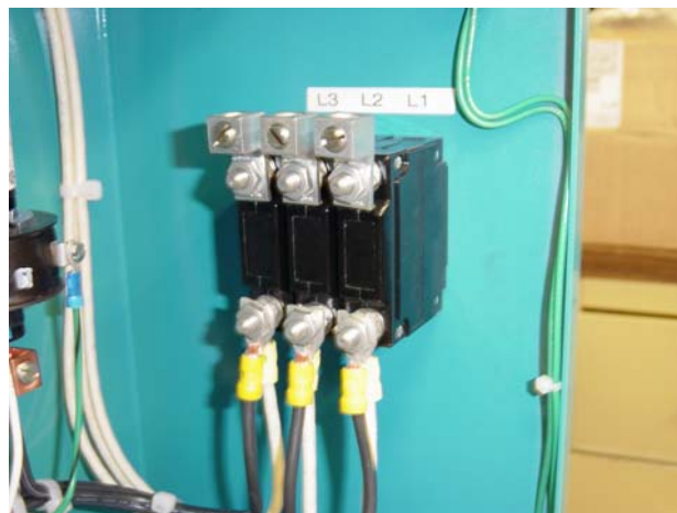
Figure 1.1 Internal view of the main breaker for connecting incoming power.
